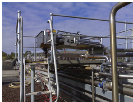
A Baleen filter installed for RAS recycle
