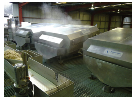
Three Baleen filters installed at a Poultry Abattoir
